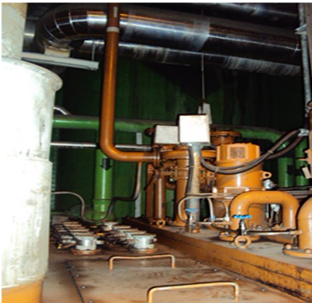
Fig. 7. Motor lube oil bfpt pump in SPP Rembang
