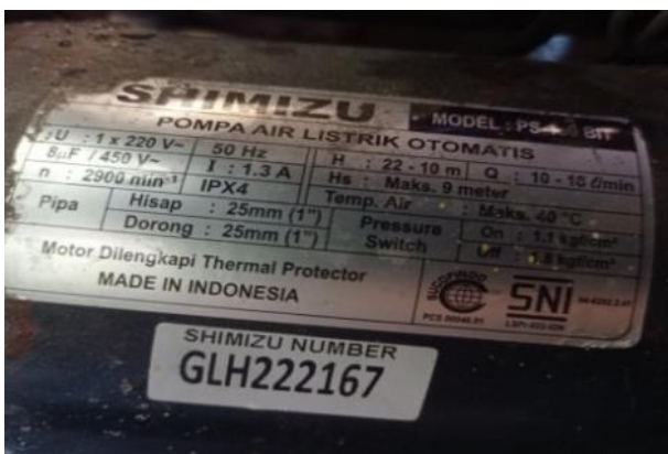
Fig. 3. Nameplate water pump
