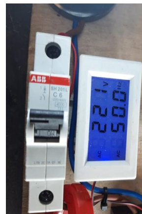
Fig. 6. AC MCB With Voltage And Current Meters
