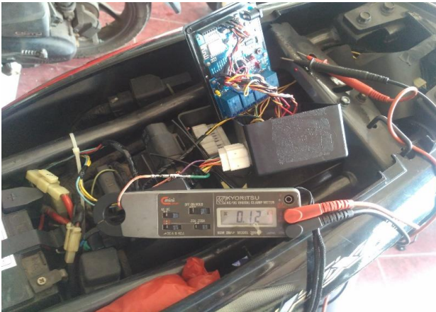
Fig. 11. Current measurement when the device installed
