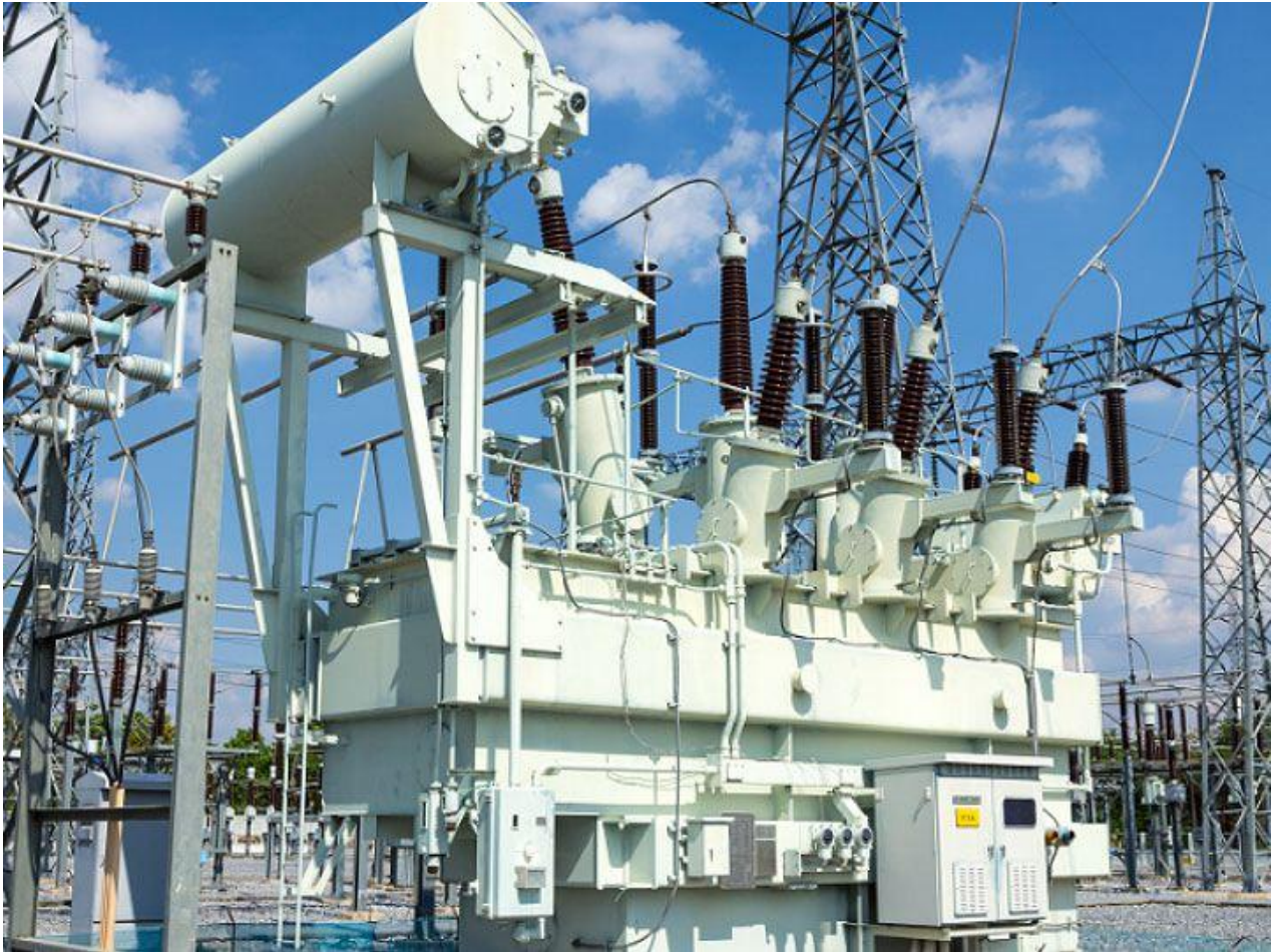
Figure 4. Power transformer in a substation
