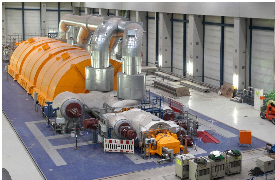
Figure 1. Power generator of steam power plant
