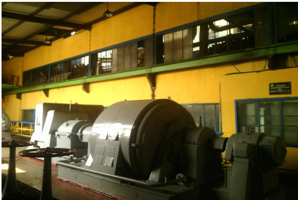
Figure 3. Steam turbine at PT Madubaru Yogyakarta, Indonesia
