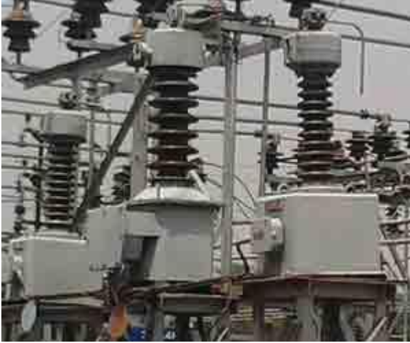
Fig. 3. Typical of voltage transformer in an outdoor substation
