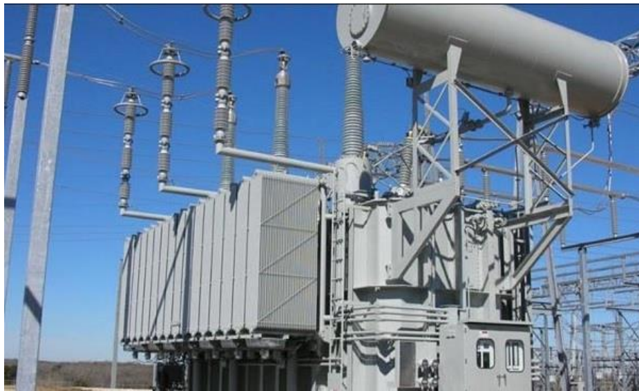
Fig. 1. Typical power transformer in an outdoor substation
