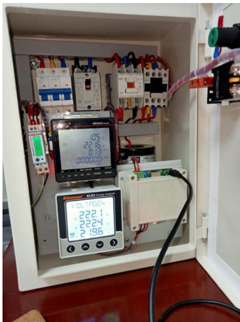
Fig. 3. The cabinet with the Modbus_Ethernet communication system for collecting, storing data, and monitoring electrical power consumption, temperature, and humidity parameters
