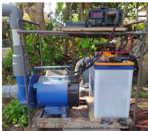
Gambar 3. Tampak Water Pump Solar Energy
