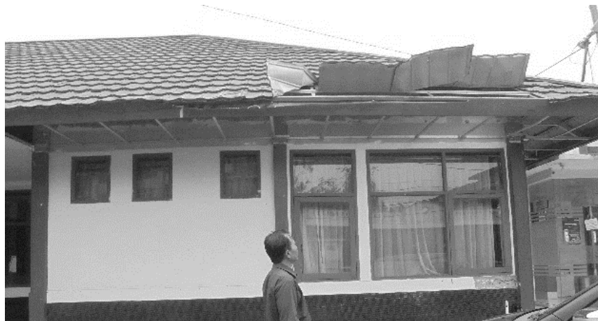
Figure 3. The right roof and ceiling cover came off.
