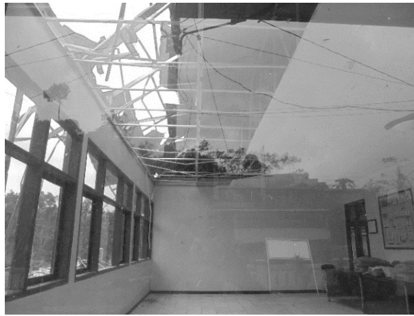
Figure 6. The gypsum ceiling cover fell
