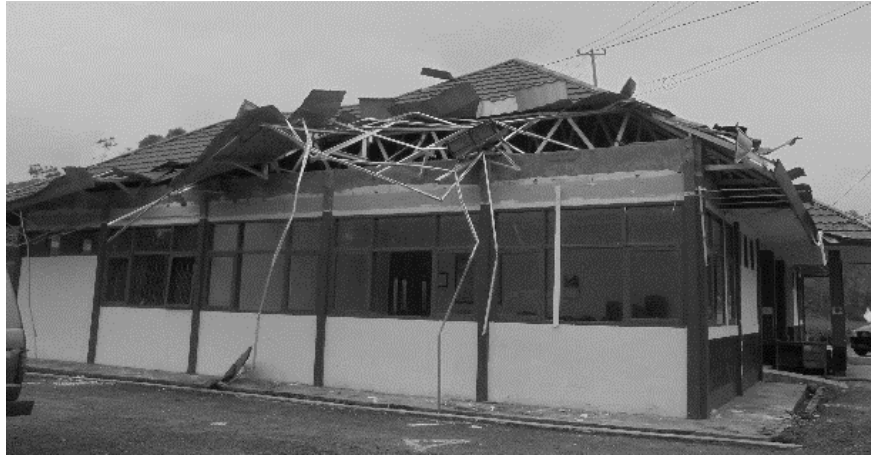
Figure 2. The roof frame of the side of the building was damaged.
