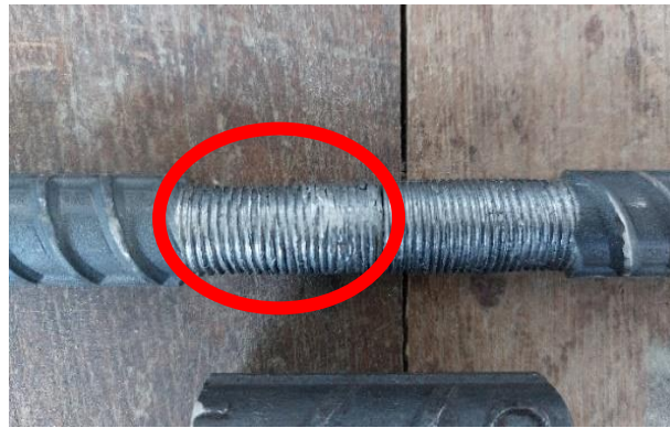
Figure 13. Damage to the thread connection
